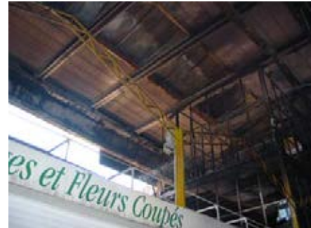
Figure CS10.2: The damaged interior of the warehouse, which was quickly repaired. (Courtesy CIMbéton, France)
